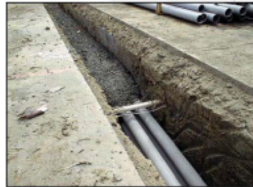
Outdoor: Concrete Encased Duct Bank
